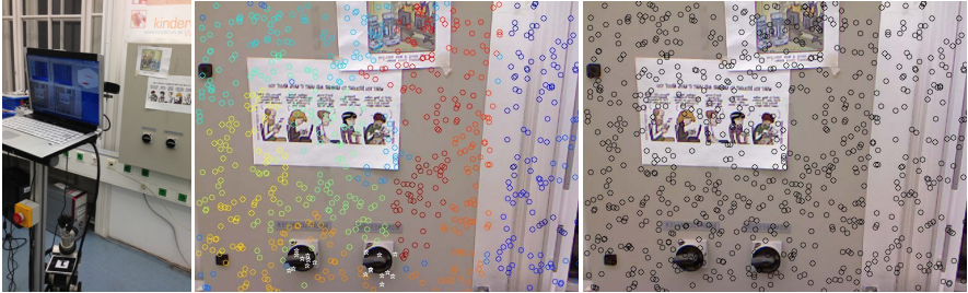
(b) Circuit breaker panel on the wall
