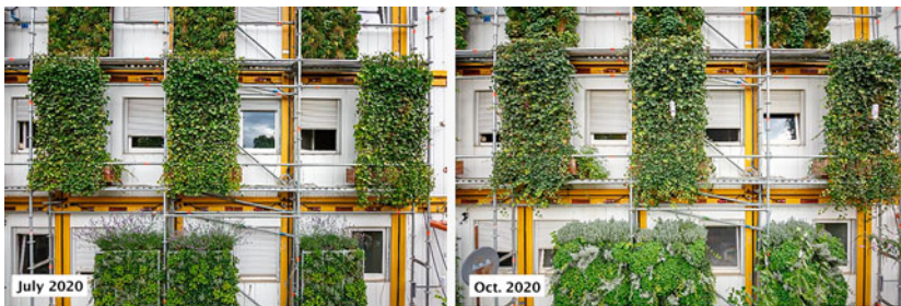
Fig. 7.3 Vertical greening of the Impulse Project Stuttgart, instant effect, due to pre-cultivation. (Photos: J. Rettig)
