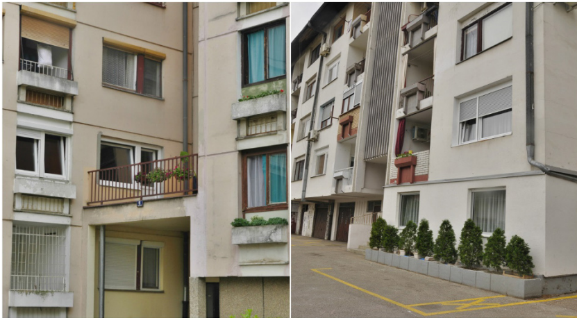
Fig. 2 Roof of building entrance appropriated for the purpose of construction of a personal terrace (left); for the purpose of gaining additional personal living space, homeowner-occupied and physically enclosed common space in the building (right). Photo by the author.
