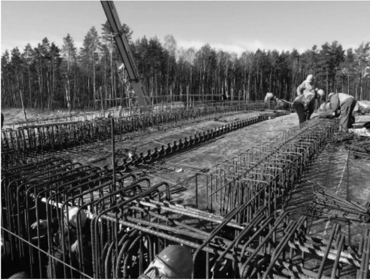
Figure 17: Reinforcement of the main girders and crossbeam (fit in reinforcement of pillars) prepared in their final position
