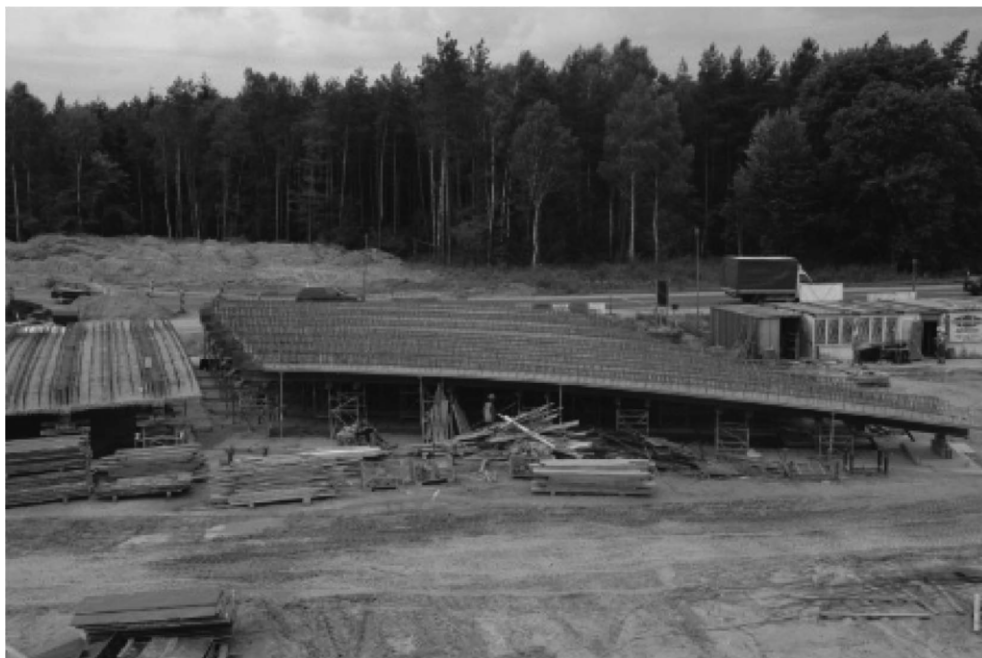
Figure 32: General view of prefabricated girders for fan-shaped span of PE1 (right) and straight girders for simple spans (left)
