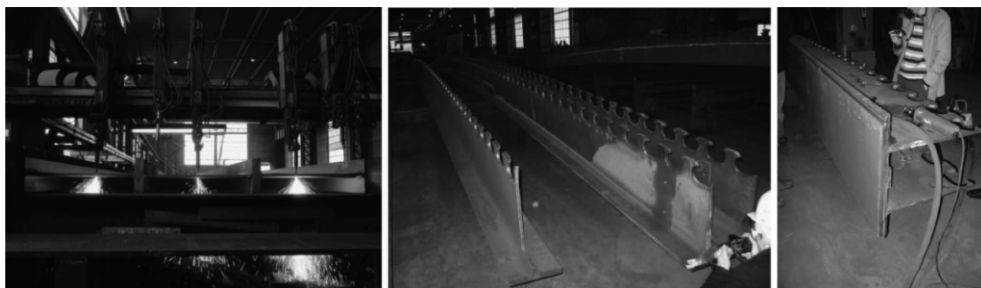
Figure 12: Fabrication of steel structure: a) separation of HEB1000 sections, b) single T-shape and tandem shape, c) additional coverplate welded at support region
