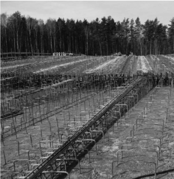
Figure 18: First concrete slab of the main girders prepared in their final position
