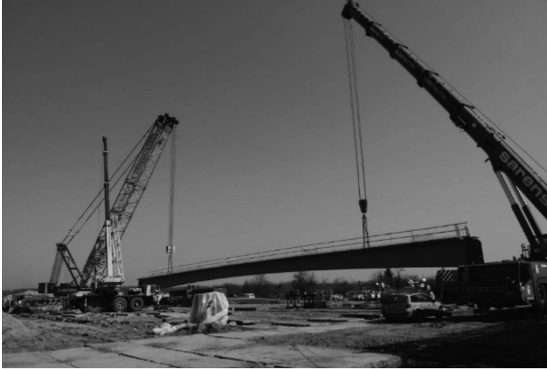
Figure 9: Using two cranes for lifting of a prefabricated girder of 63 m frame on Route Sucharskiego
