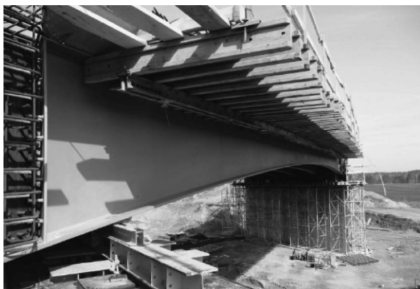
Figure 15: Additional scaffolding of external beam and constant thickness of bottom flange is visible.
