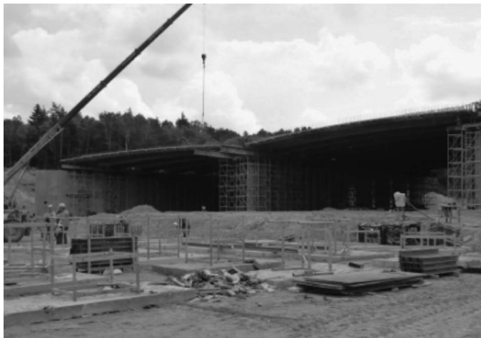
Figure 22: The prefabricated girders of the second line of PE4 structure in their final positions
