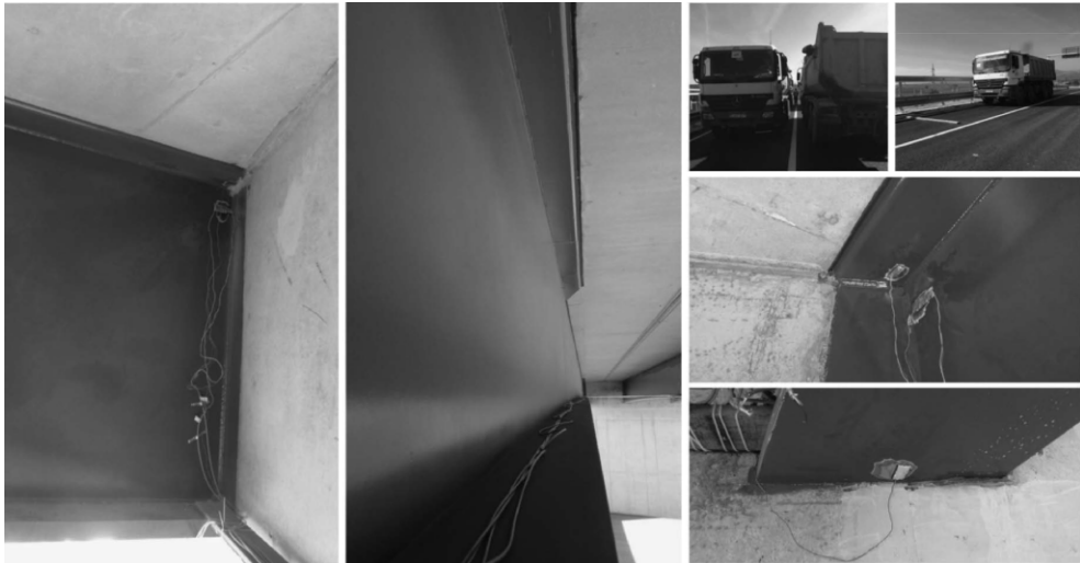
Figure 14: Installed strains on the section of the bridge in the in-situ test day
