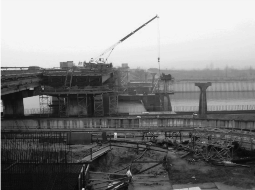
Figure 42: The crane on prefabricated VFT girders operating on the pillar of neighboring pedestrian bridge under construction
