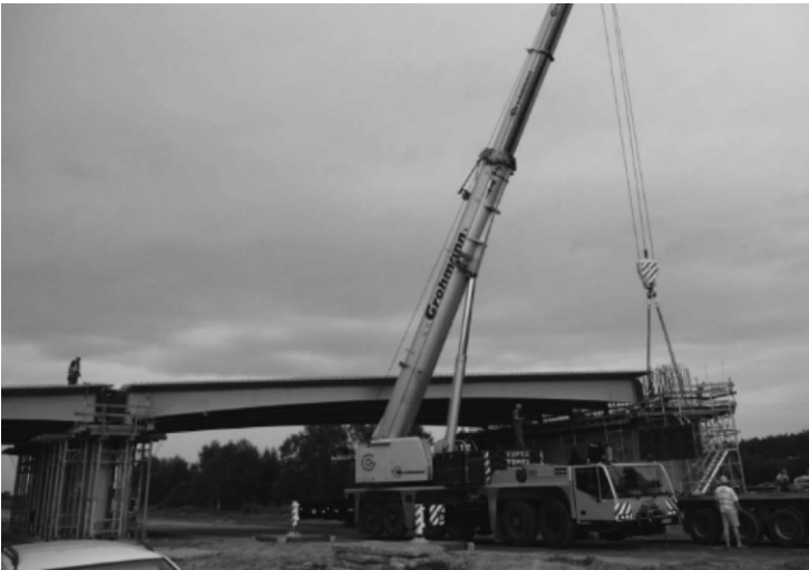
Figure 14: Montage of typical solution of overpass at S7 road – 2 span VFT integral bridge – directly from trucks
