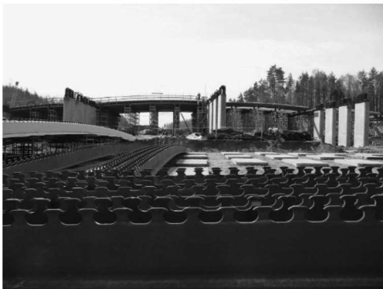
Figure 15: Steel shapes at front and girders of first line of the bridge in final position in the background
