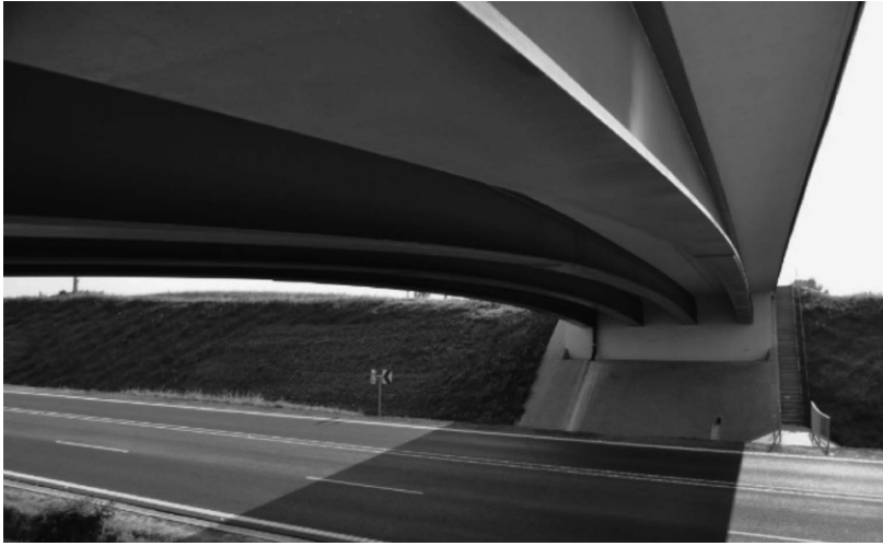
Figure 6: Bottom view of typical single span frame (VFT viaduct above bypass of Goldap)
