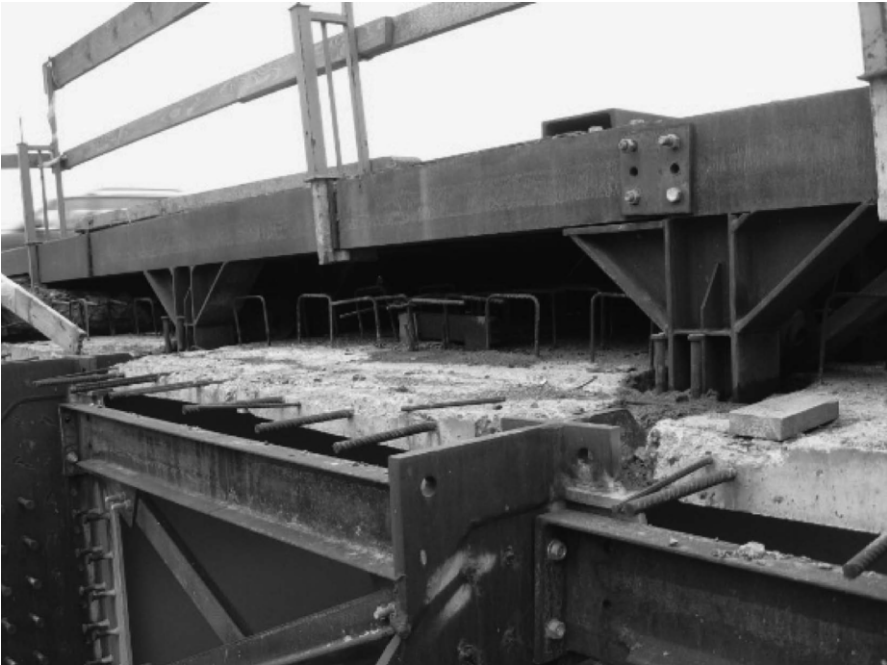
Figure 41: Special steel structure and modification of ordinary VFT solution of steel girders for temporary support of crane
