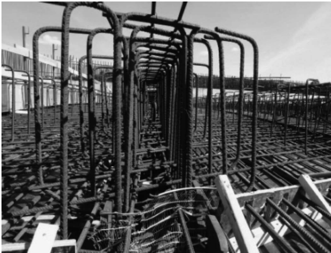
Figure 21: Realized reinforcement system of A4 beam for side span of PE4 structure
