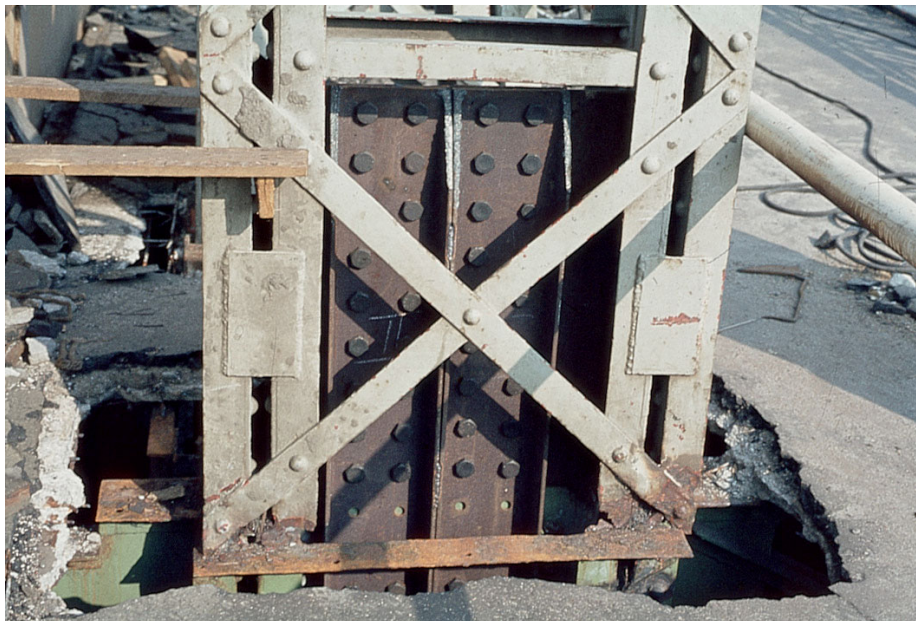
Figure 12: Temporary strengthening of the collapsed member
