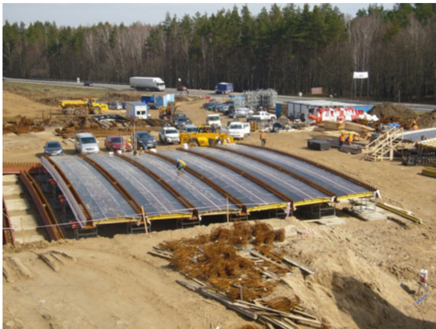
Figure 6: Fabrication area to cast the prefabricated elements next to the construction site
