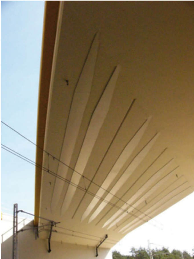
Figure 12: Bottom view on the external reinforcement of bridge WD-4 which adapts the force flow
