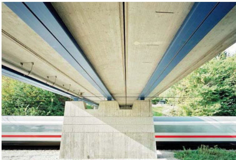
Figure 4: Bottom view with three VFT-WIB girders and spring plates at the middle support
