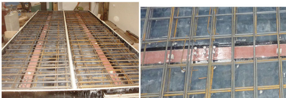
Figure 9: Composite truss before concrete casting and the detail of the connection above the node
