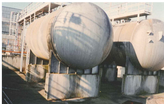
Figure 2: Horizontal cylindrical reservoirs resting on saddles of support
