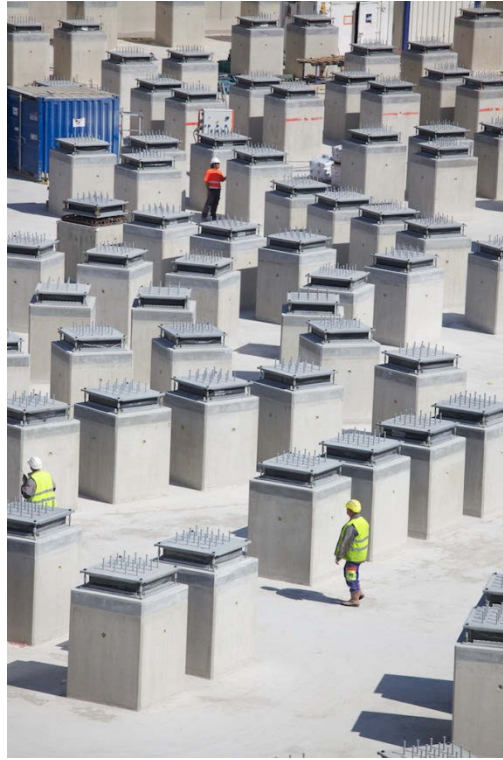
Figure 8: Fan-shaped arrangement of the seismic isolation system under the cryostat and Tokamak machine supporting structure
