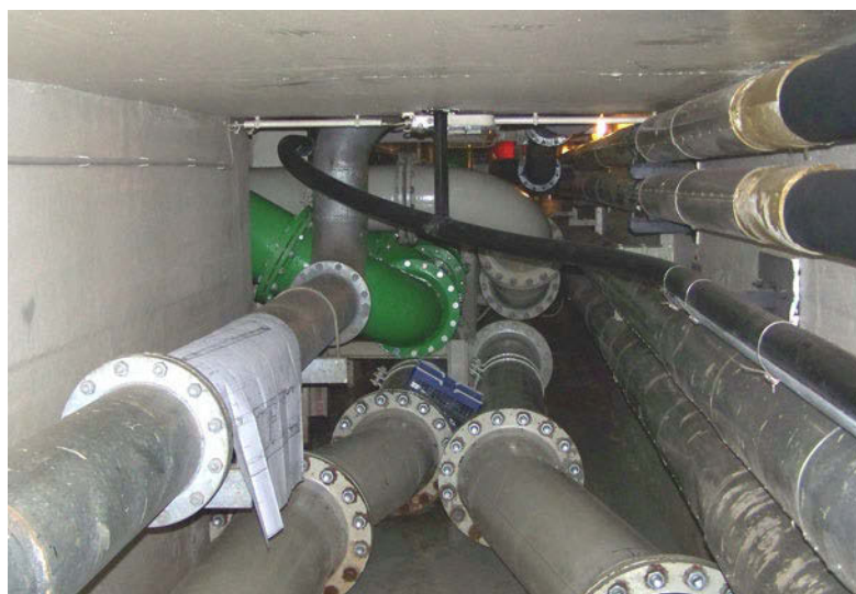
Figure 1: Because of obstructed access, pipes had to be shut off and removed
