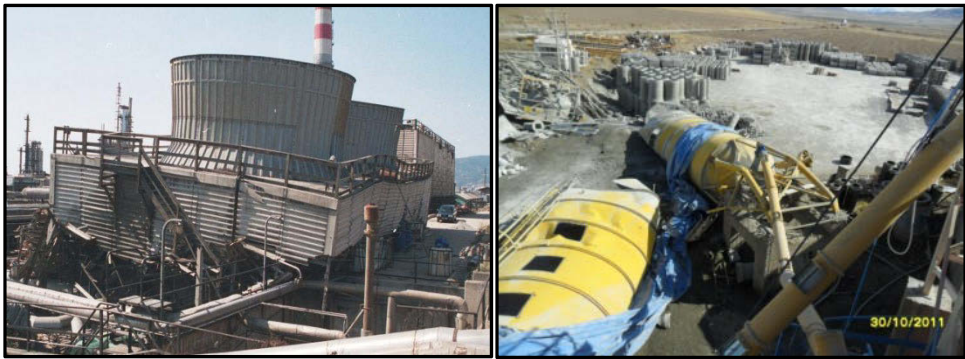
Figure 6: Collapsed silo at SEKA Factory in Izmit (left) and cement silo in Van
