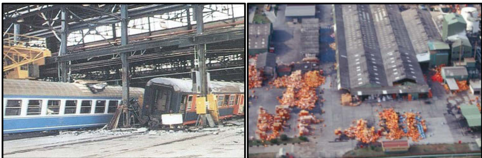
Figure 4: Damaged steel structure at Adapazari rail car factory (left) and losses of open stored materials
