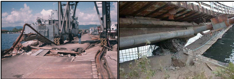
Figure 7: Damage at navy port in Gölcük (left) and failed column at SEKA port
