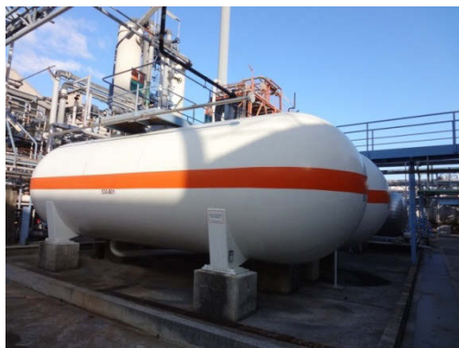
Figure 1: Horizontal cylindrical reservoirs resting on four legs system support
