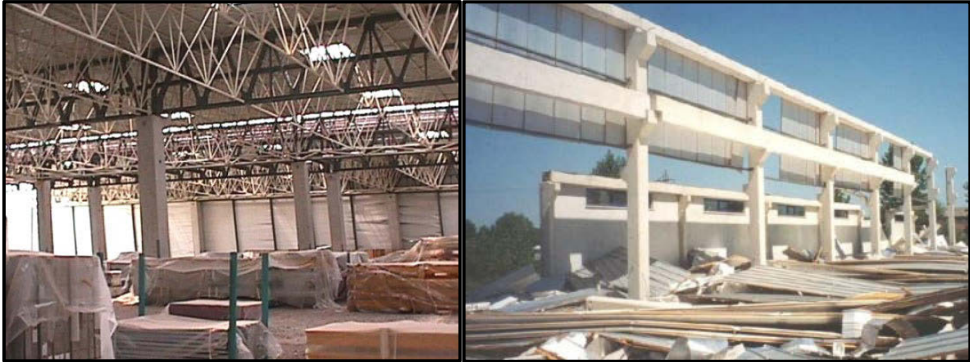
Figure 3: Damaged prefabricated buildings at Ford Otosan Plant
