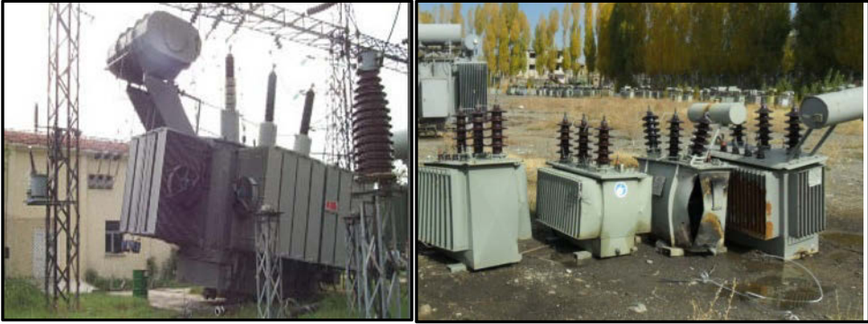
Figure 5: Damaged transformers at Izmit substation (left) and in Van
