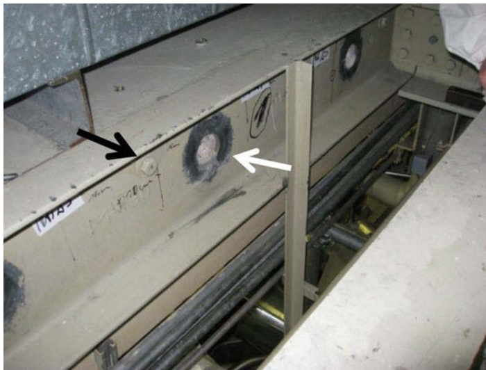
Figure 6: Replacement of Liebig Anchors, technical approval of 1975 (black arrow), by Hilti HDA Anchors, technical approval of 2008 (white arrow)
