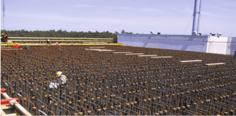
Fig. 17.1 Reinforcement of the roof of the Vitrification Facility Karlsruhe (Ger.: VEK)—the load case airplane crash is the design basis for the massive reinforcement
