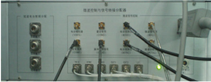
Fig. 30.4 Latest microwave test in ATDS passing through microwave controller
