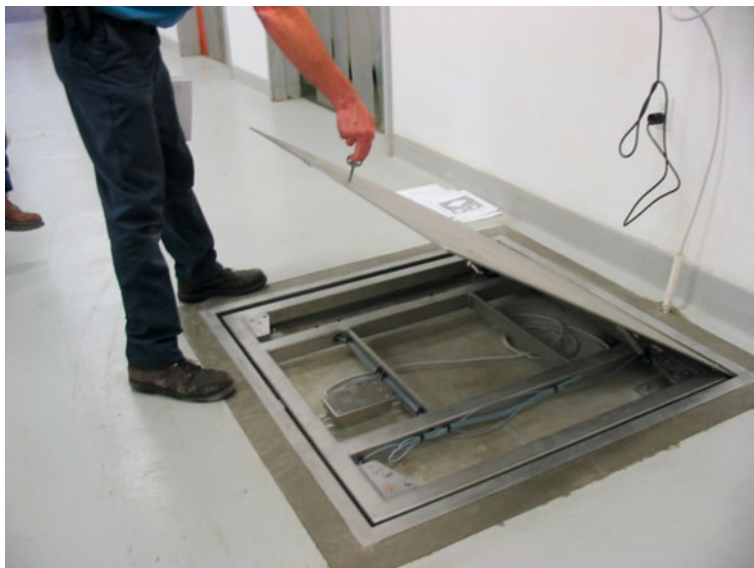
Fig. 3 Sartorius pit-mounted scale, flush with the floor, platform lifted for cleaning
