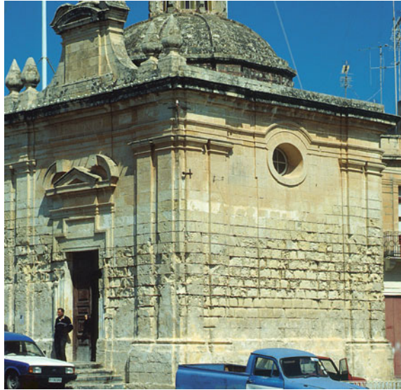
Fig. 4.17 Sea-salt-induced deterioration at Santa Marija Ta' Cwerra church (Malta); Photo: B. Fitzner, Geological Institute, RWTH Aachen University
