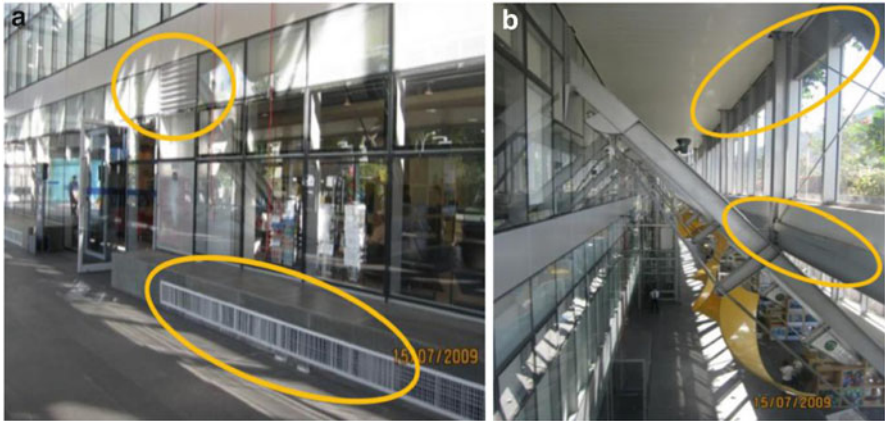
Fig. 8.6 Supply, return air vents, and top shutter: (a) supply and return air vents and (b) top shutter
