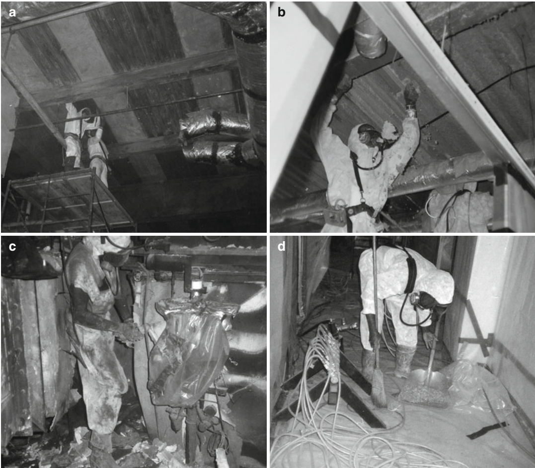
Fig. 2.4 Workers in the North Carolina asbestos-abatement program. Asbestos removal occurs within confined spaces. Note the respiratory equipment and special protective clothing
