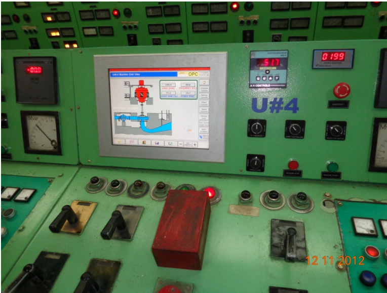
Fig. 2. Control Room Panel of a Hydropower Plant
