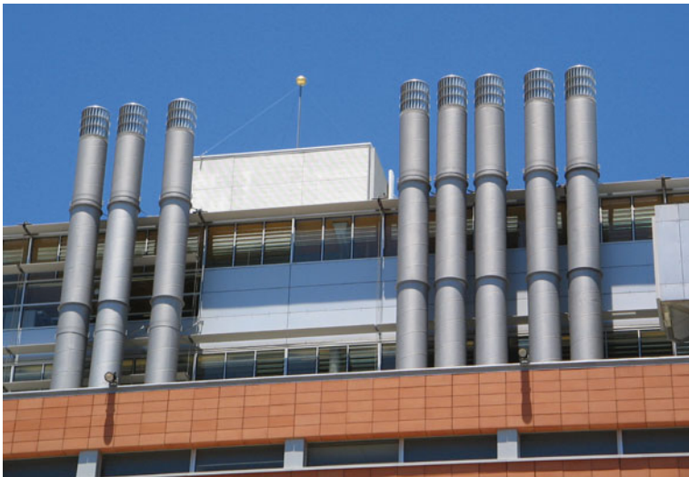
Fig. 11 Cylindrical centrifugal ventilator at the University of New South Wales
