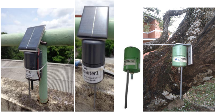
Fig. 5. The RTU (left) and a Repeater (right)
