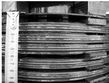
Fig. 6. Transformer winding with deformation D2 – top two discs lowered to minimum
