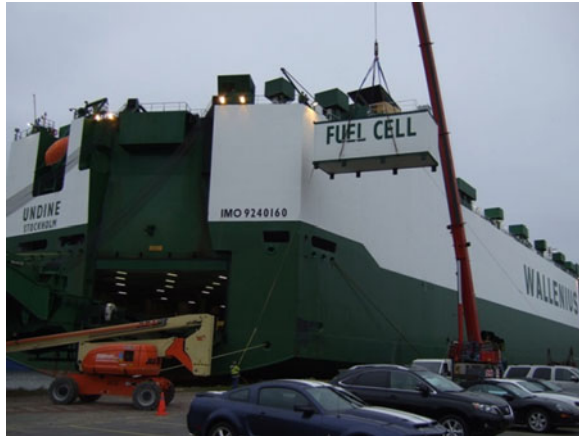
Fig. 6.143 Installation of the Wärtsilä WFC20 fuel cell unit on-board of the “Undine” of the Swedish Wallenius Lines
