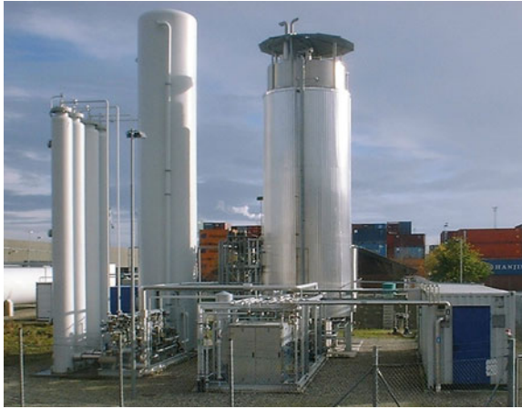
Fig. 6.101 Caloric HM methanol steam reforming plant with a hydrogen capacity of 750 Nm 3 /h [541]
