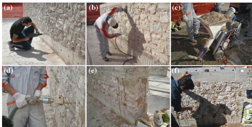
Fig. 8 Grout injection on stone masonry walls [4]: a drilling holes for the injection; b cleaning the drilled holes by blowing compressed air; c injection pump machine; d injection of a wall; e grout mixture leaking from a “control” hole; f sealing of the hole with mortar
