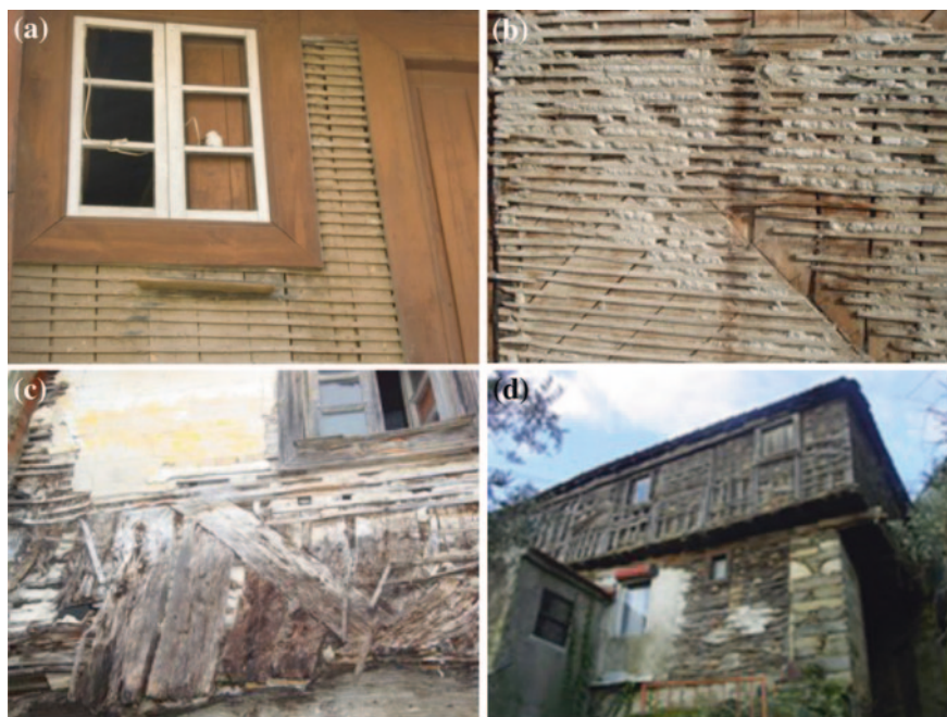
Fig. 2 Timber structural system typologies of tabique walls. a Typology 1. b Typology 2. c Typology 3. d Typology 4
