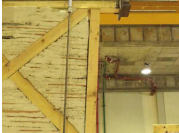
Fig. 13 Detachment between the masonry filling and the Gaiola structure [12]
