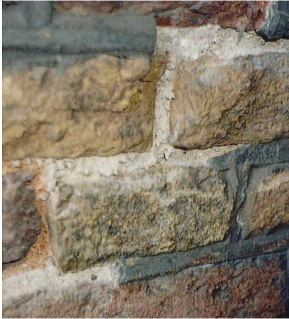
Fig. 7 Push-out of cement re-pointing due to crystallization of salts at the interface of new pointing and old bedding mortar
