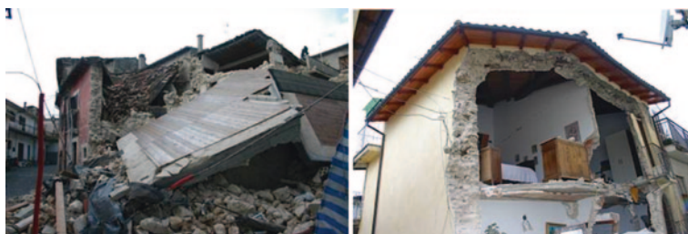
Fig. 7 Damage caused by past interventions, Abruzzo 2009
