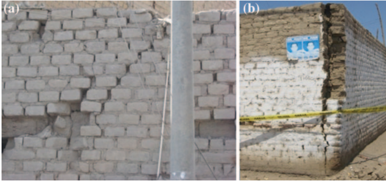
Fig. 20 Typical crack patterns in adobe masonry walls. a Stair crack shape (concentrated on mortar). b Vertical crack (fracture of bricks)
