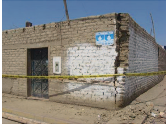
Fig. 7 Vertical crack at the corner of an adobe house, Pisco earthquake, Peru, 2007
