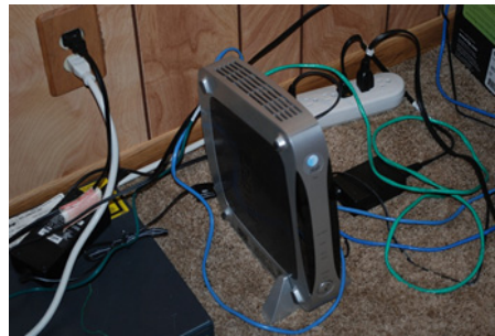
Fig. 7. Multiple wires around the router
