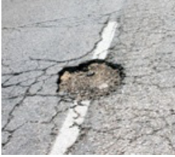
Fig. 1. Image of pothole [10]
