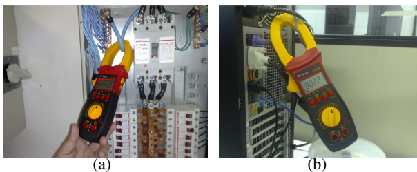
Fig. 6. Power (current) measurement setup. (6(a)) Cluster setup: the total current consumed by Enterprise 3 was measured on the neutral wire of its power distribution panel. (6(b)) BOXX Personal Supercomputer setup: the total current consumed by it was measured on the neutral wire of its power cord.
