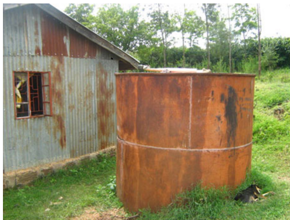
Fig. 2 Water tank 2 for domestic use
