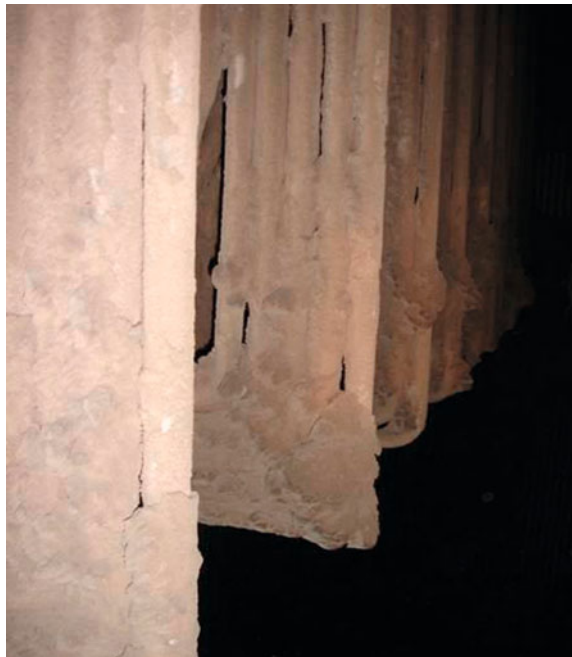
Fig. 20.3 Photo of superheater with deposits accumulated as a result of biomass combustion
