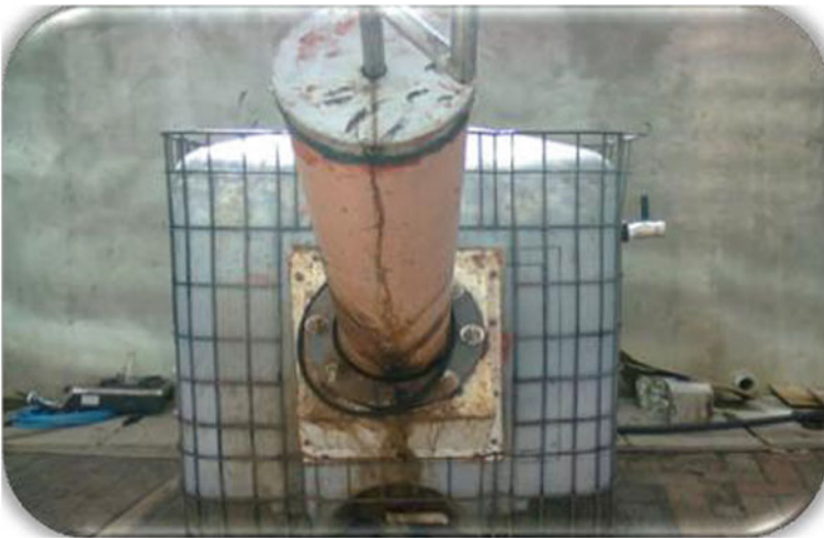
Fig. 37.4 Front view of digester
