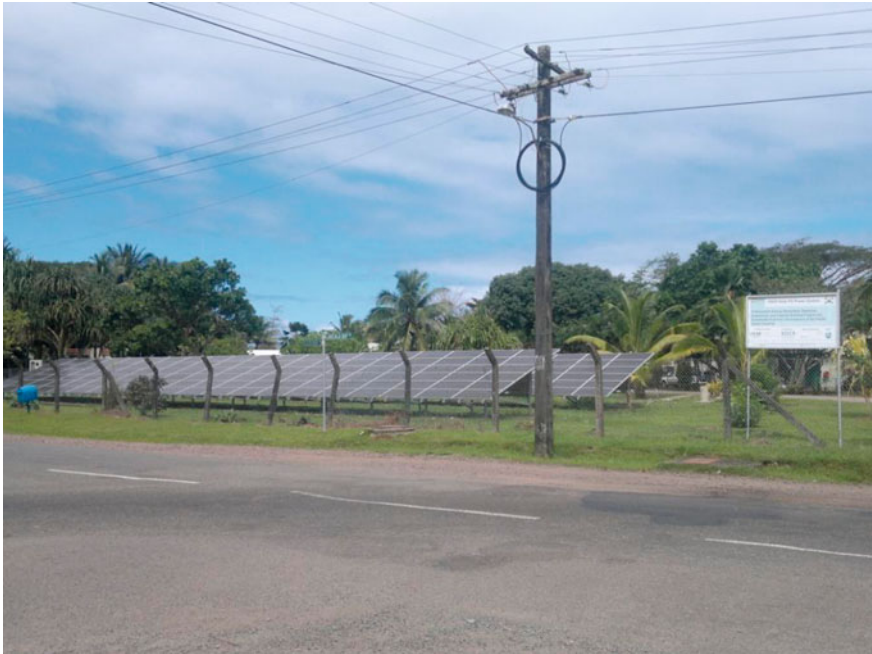
Fig. 1.2 45 kW grid connected PV system in Fiji
