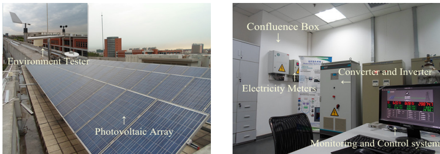
Fig. 6. Photovoltaic system owned by Department of Automation, SJTU
