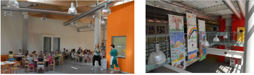
Fig. 5. Across the building the construction, electrical and ventilation systems are left visible to show how the building functions. a) Dining area b) Entrance hall.
