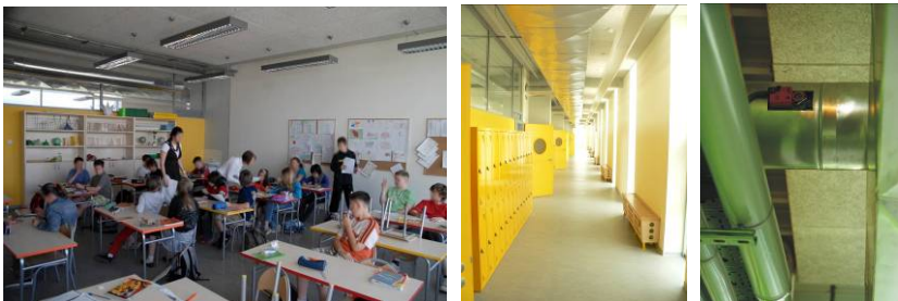
Fig. 3. a) Classroom with MV ducts visible, b) Corridor with MV ducts visible, c) Location of the control gear for MV at ceiling high
