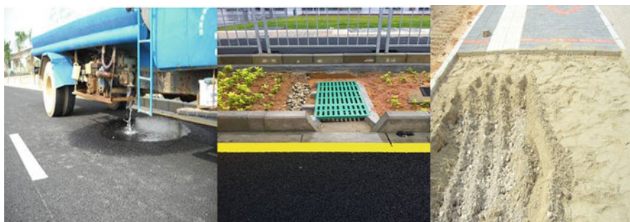
Fig. 14.2 The LID facilities in Guangming railway demonstration area
