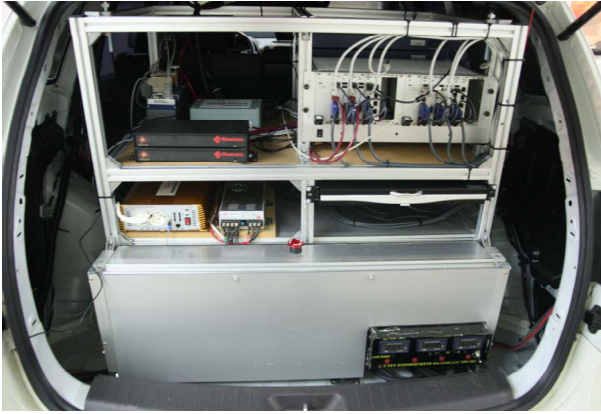
Fig. 4. Controllers and communication system in the trunk of the vehicle
