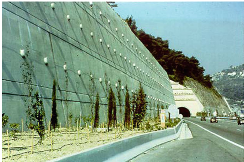
Analysis and Design Issues of Geotechnical Systems: Rigid Walls, Fig. 6 Soil-nailed walls
