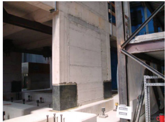
Assessment and Strengthening of Partitions in Buildings, Fig. 7 CFRP reinforcement of the column to safeguard against lap-splice failure (Chrysostomou et al. 2014 with kind permission from Springer Science and Business Media)
