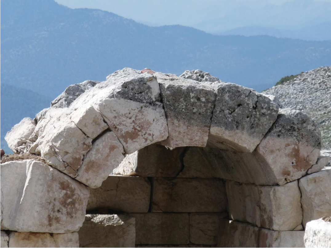
Archeoseismology, Fig. 7 A dropped keystone in the Roman Baths at Sagalassos (SW Turkey), interpreted as a potential earthquake archeological effect (cf. Similox-Tohon et al. 2006) © Sintubin
