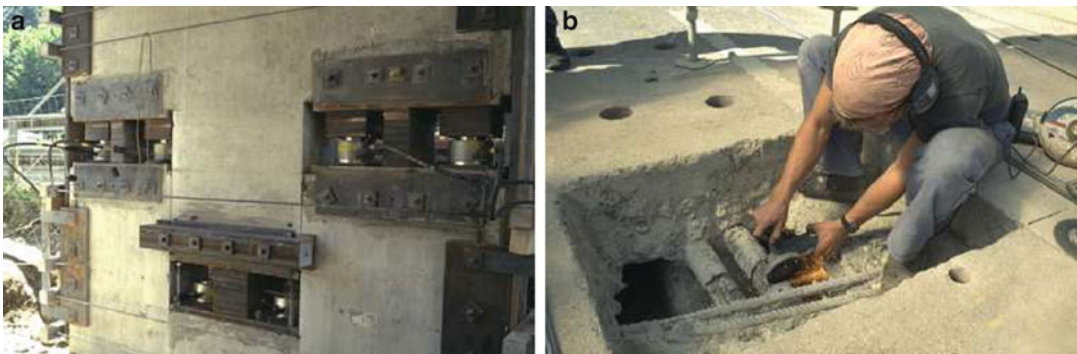
Vibration-Based Damage Identification: The Z24 Bridge Benchmark, Fig. 2 Settlement system used for damage scenarios 3–6 (a) and cutting of tendons for scenarios 15–17 (b)
