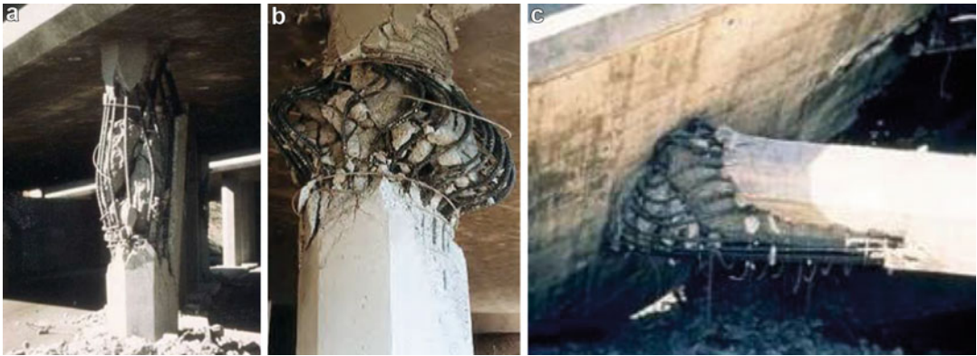
Strengthening Techniques: Bridges, Fig. 5 Column shear damage (© California Department of Transportation (2006))
