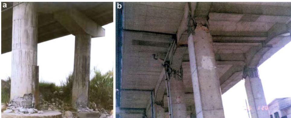
Strengthening Techniques: Bridges, Fig. 4 Column flexural damage (© California Department of Transportation (2006))
