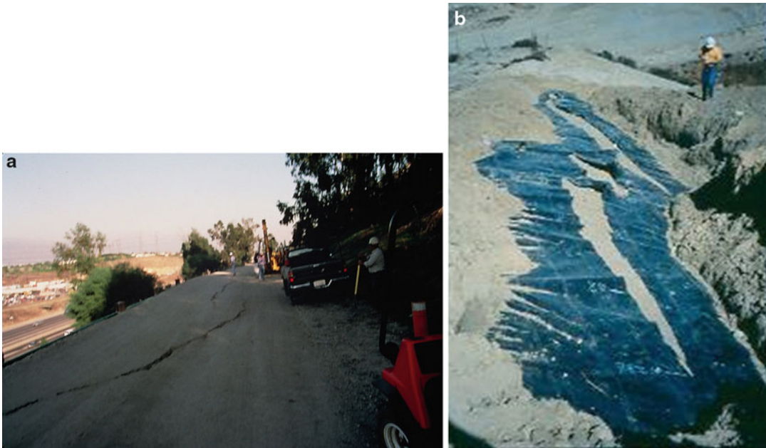
Seismic Design of Waste Containment Systems, Fig. 2 Damage to landfills observed following the Northridge earthquake: (a) cracking in soil cover on the
