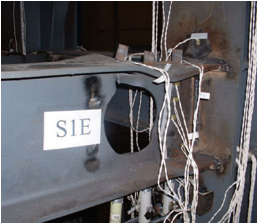
Strengthening Techniques: Code-Deficient Steel Buildings, Fig. 5 Failure mode of connection with circular web opening (Qingshan et al. 2009)
