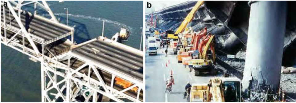
Strengthening Techniques: Bridges, Fig. 1 Bridge failure: (a) San Francisco-Oakland Bay Bridge (© California Department of Transportation (2003)
