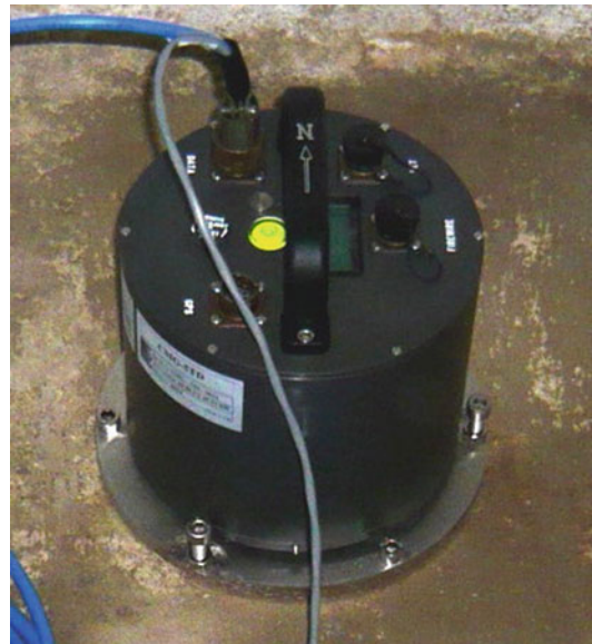
Seismic Accelerometers, Fig. 15 CMG 5TD from Güralp Systems. This model can include a recorder and an Ethernet interface. The photo shows a unit installed in an underground gallery with the mounting base anchored to the concrete ground
