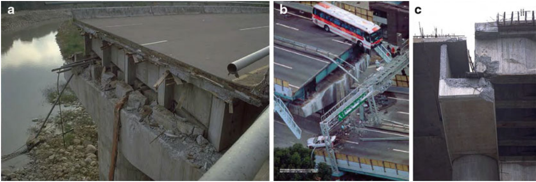
Strengthening Techniques: Bridges, Fig. 2 Deck failure: (a), (b) span collapse (© California Department of Transportation (2006)); (c) span displacement
