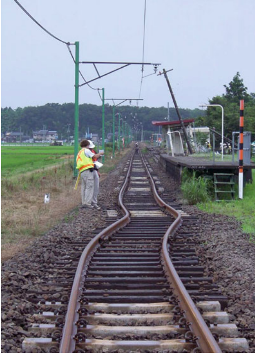
Seismic Vulnerability Assessment: Lifelines, Fig. 3 Lateral deformation of train tracks at the Arahama station due to surface waves in 2007 Niigata-Chuetsu Oki ( M_w 6.6) earthquake (Photo Credit: US Geological Survey)
