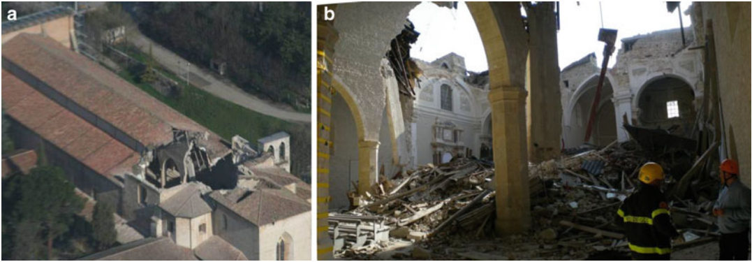
Seismic Behavior of Ancient Monuments: From Collapse Observation to Permanent Monitoring, Fig. 1 Basilica of S. Maria di Collemaggio transept collapse: (a) aerial view and (b) internal view
