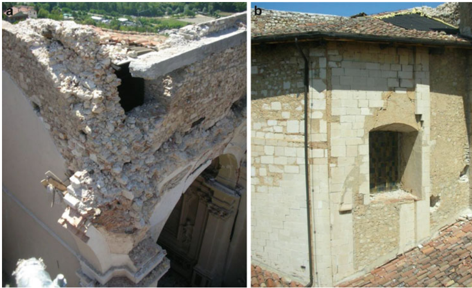
Seismic Behavior of Ancient Monuments: From Collapse Observation to Permanent Monitoring, Fig. 3 Masonry features at L'Aquila: (a) masonry quality
