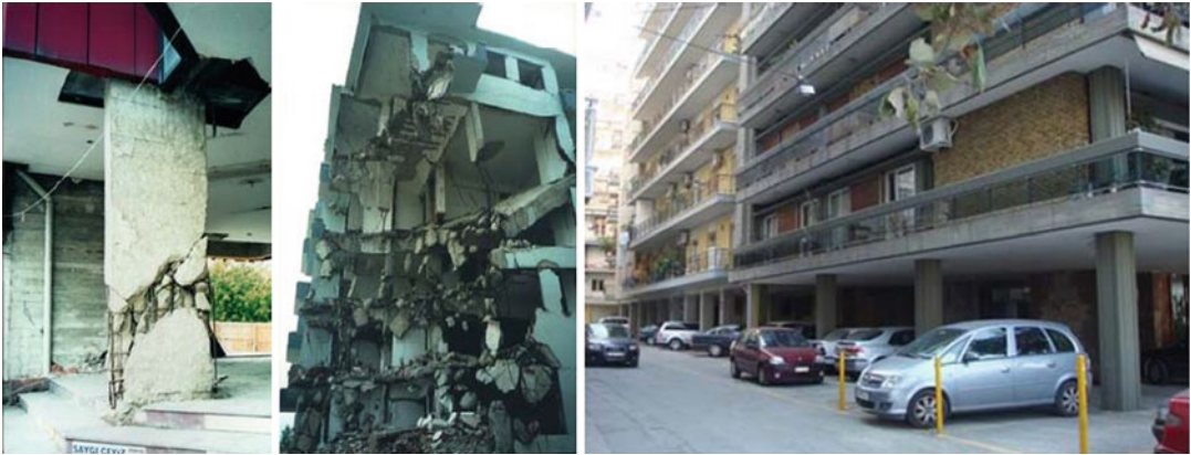
Strengthened Structural Members and Structures: Analytical Assessment, Fig. 1 Damage patterns in old-type R/C members and structures; typical multistory R/C residential buildings with pilotis in Greece (Source of figures: author's personal files)
