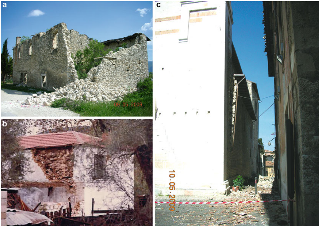
Strengthening Techniques: Masonry and Heritage Structures, Fig. 13 (a) collapse of the corner of a building, (b) partial collapse of the exterior leaf of
