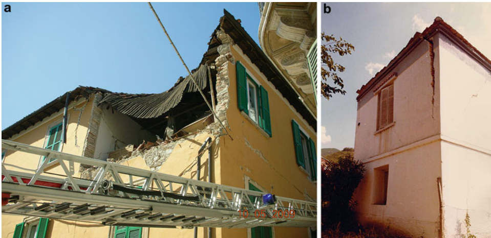
Strengthening Techniques: Masonry and Heritage Structures, Fig. 15 Typical damages due to out-of-plane bending of walls
