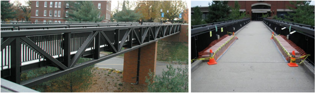
System and Damage Identification of Civil Structures, Fig. 1 Dowling hall footbridge ( left ) and placement of concrete blocks on the bridge ( right )
