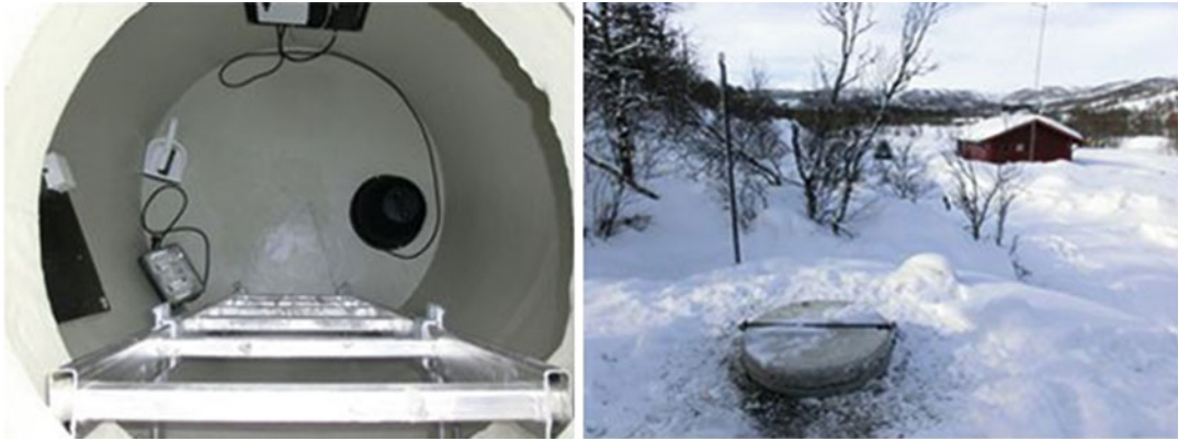
Seismic Network and Data Quality, Fig. 5 Example of a seismic station installed in southern Norway. The vault housing (with the seismometer and digitizer) is constructed from prefabricated concrete rings. ( left ).
