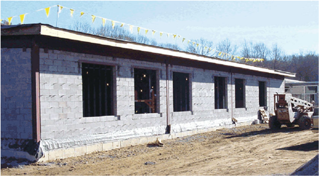
Strengthening Techniques: Code-Deficient Steel Buildings, Fig. 19 Ordinary hybrid wall (Adopted by http://masonryedge.com/site/mim-archives-the-storypole-vol-38-no-4/143-filling-in-the-frame- )
