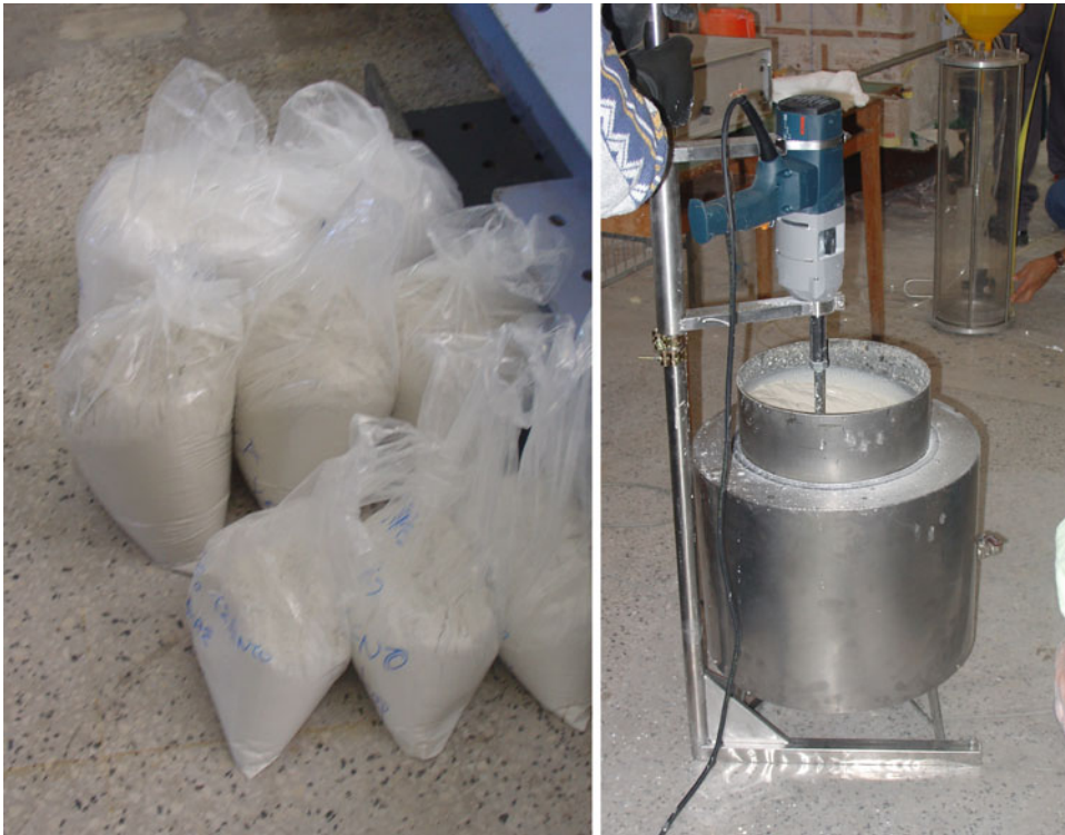
Strengthening Techniques: Masonry and Heritage Structures, Fig. 10 Materials for preparation of the grout mix. High turbulence mixer
