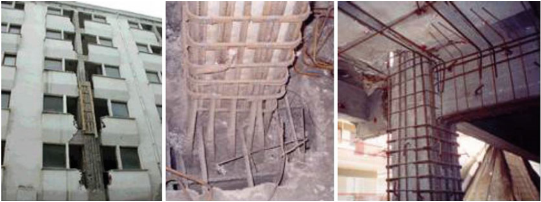
Strengthened Structural Members and Structures: Analytical Assessment, Fig. 7 Column R/C jacketing (Source of figures: author’s personal files)
