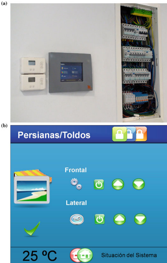
Fig. 6 Control panel prototype. a Control panel installed in the reference building. b HMI of the integrated software
