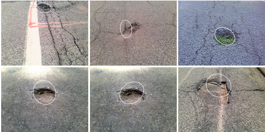
Fig. 9. Detection of asphalt pavement potholes
