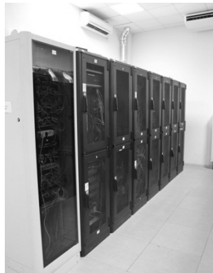
Fig. 2. Front side of racks
