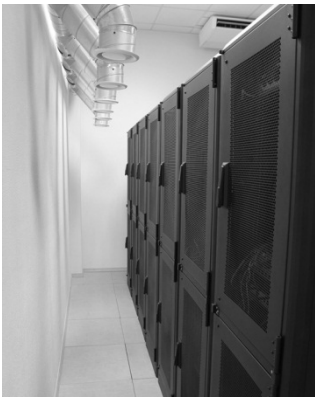
Fig. 1. Back side of racks
