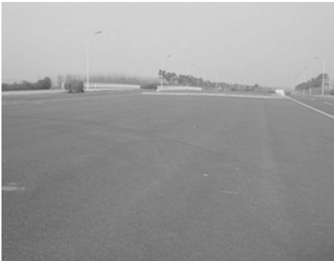
Plot 4 AMFM Field Test Site on Site
