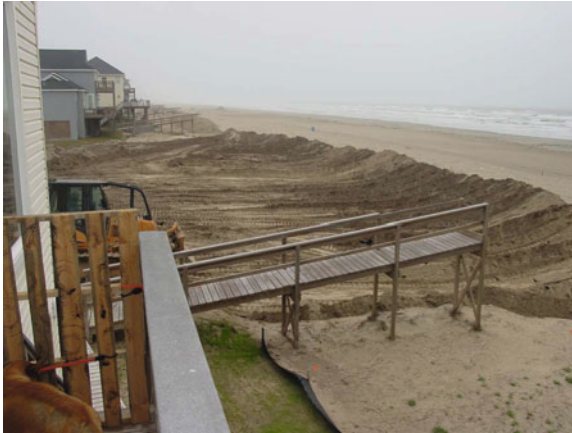
Fig. 6.4 Digging out the swale and reconstructing the foredunes, Sandhill Shores project. The reconstructed locations of the dune, swale, and their heights/depths were marked on flags for the bulldozer operator to follow. The dune was reconstructed after the storm with the aid of a GIS, GPS, and survey equipment, but the dimensions and volume were defined to match pre-storm topography, as based upon a LIDAR elevation dataset and aerial photography taken before the storm. Photo by Paul White
