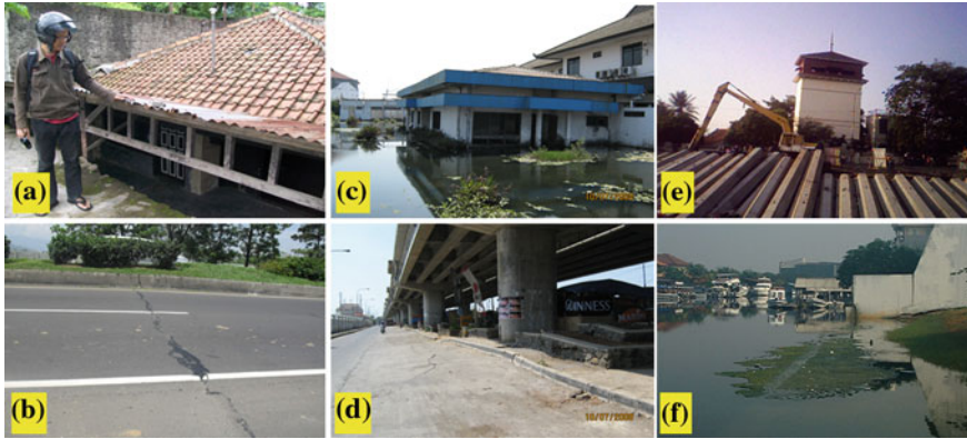
Fig. 2 Examples of subsidence impacts in urban areas, after Abidin et al. [7–9]. a Subsided house in Bandung; b highway cracking in Bandung; c abandoned building in Semarang; d cracking in highway infrastructure and bridge in Semarang; e tilted building in Jakarta; f coastal flooding in Jakarta
