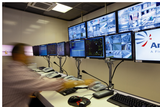
Fig. 1. Control room for the security management system
