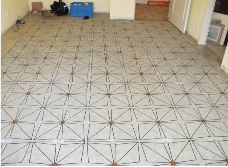
Fig. 9. SensFloor underlay installation under progress at the assisted living apartment, which floor plan is depicted in Fig. 12 (living room, corridor). The underlay has four radio modules and 32 sensor areas per square meter.
