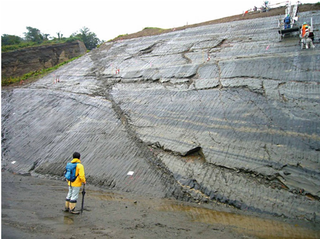
Photo. 14.3 Fault appeared on the cut-slope
