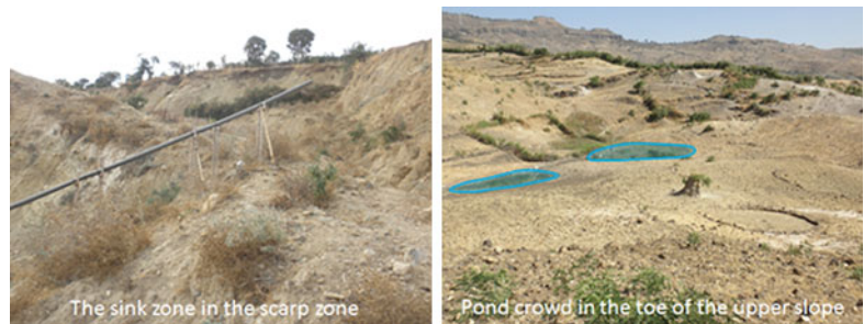
Photo 42.4 Landslide situation in L/S28 site
