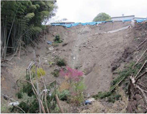
Fig. 59.4 Landslide in Kami-Kashiwazaki district (a)
