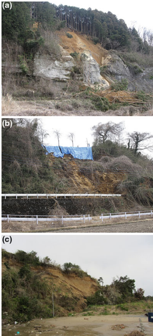
Fig. 58.6 a Surface failure in Utsunomiya city, in Tochigi prefecture.tif. b Surface failure in Nakagawa town, Tochigi prefecture.tif. c Surface failure in Hitachi city, Ibaraki prefecture.tif
