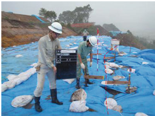
Photo 33.4 Vertical drops appeared on the BB' cross section
