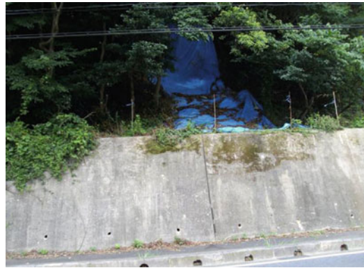
Fig. 93.9 Small slope failure in July 2009
