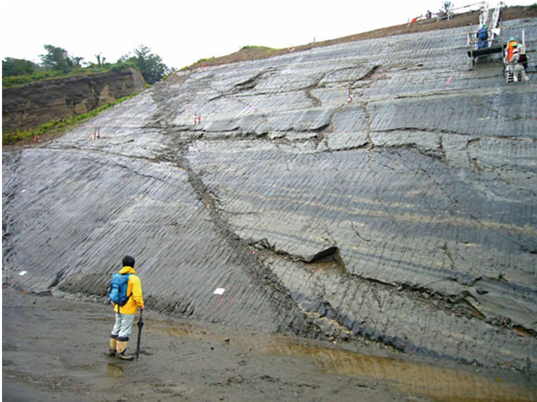
Photo. 14.3 Fault appeared on the cut-slope
