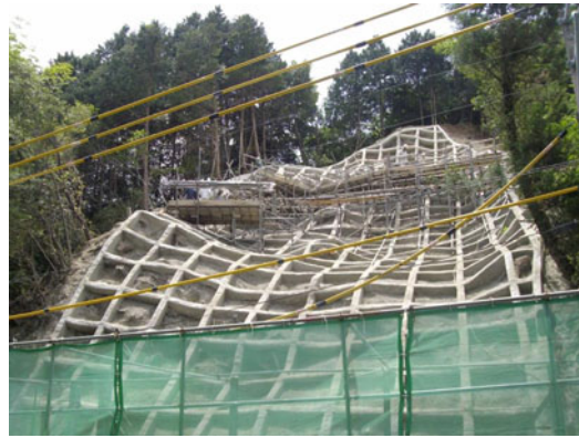
Fig. 93.8 Slope protection works on the end of extrapolation of active fault estimated \gamma -ray measurement
