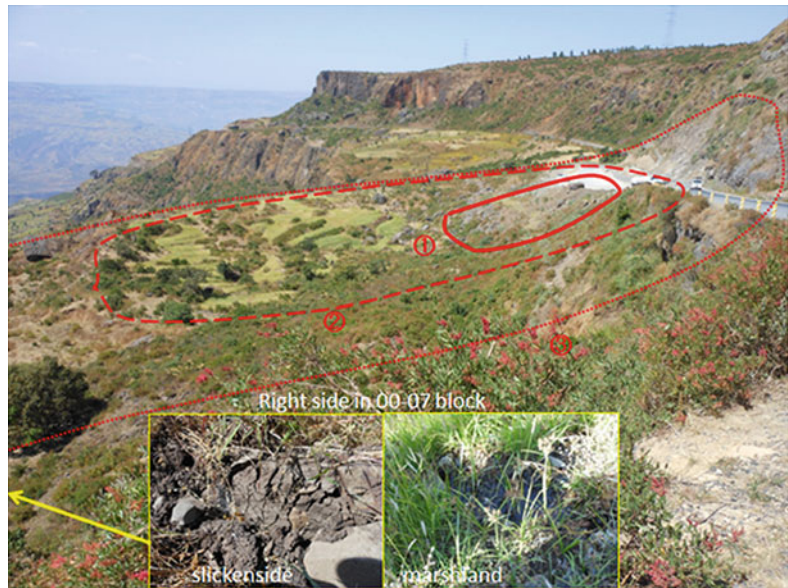
Photo 42.1 Landslide situation in L/S00 site
