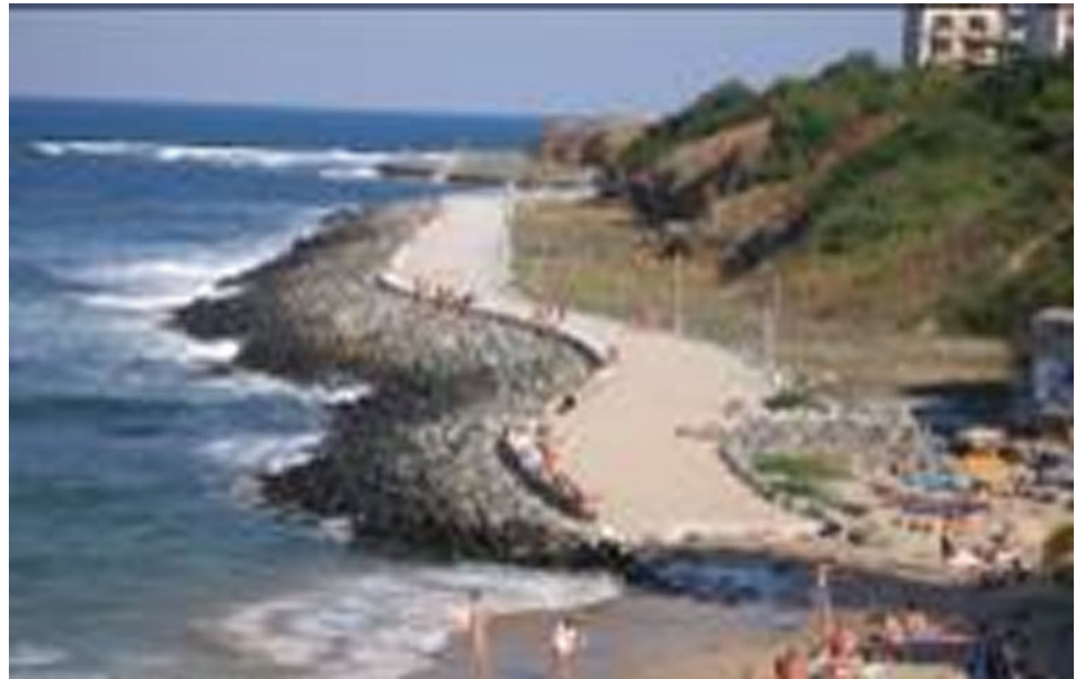
Fig. 9 The same section of the coast north of Primorsko after the construction retaining structures
