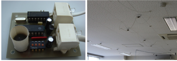
Fig. 1. The sensor module and the interconnection of sensor nodes with cables
