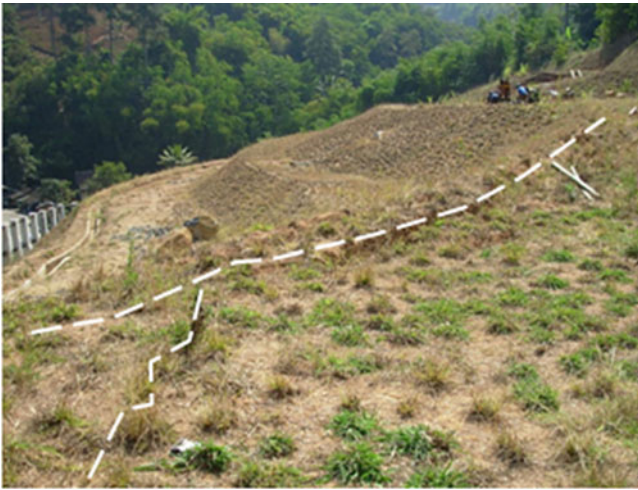
Fig. 1 Research slope located above the Cadas Pangeran Provincial Road, Sumedang District, West Java, Indonesia. Dashed white lines indicate tension cracks (Photograph was taken on May 2006)
