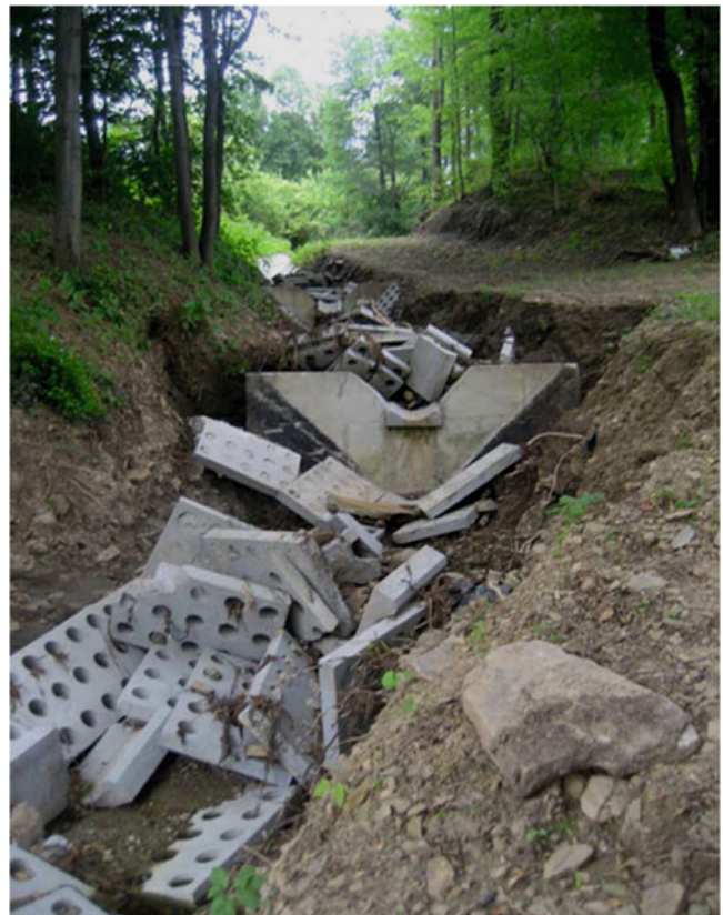
Fig. 10 Damages of drainage system – landslide no 6
