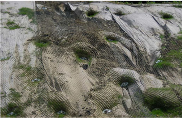
Fig. 6 Damages in partly stabilized lower part of landslide no 1
