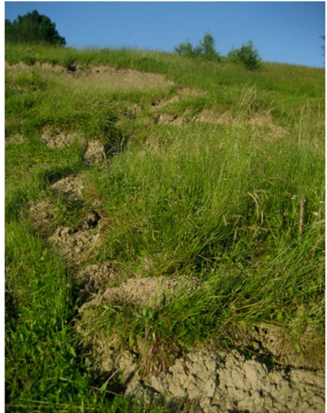
Fig. 9 New cracks – land no 5
