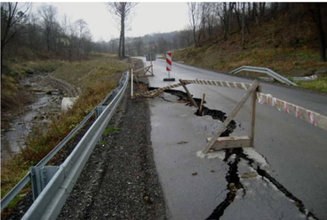
Fig. 8 Destructions of a public road (erosion) landslide no 6
