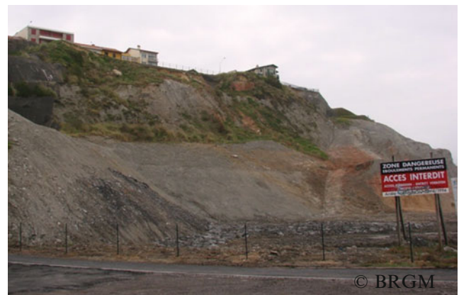
Fig. 9 Forbidden area due to frequent landslide occurrence on the South of the Côte des Basques (see localisation on Fig. 10)
