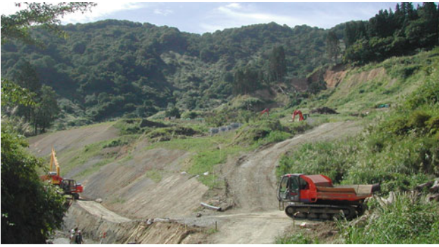
Photo 1 Overview of the landslide site
