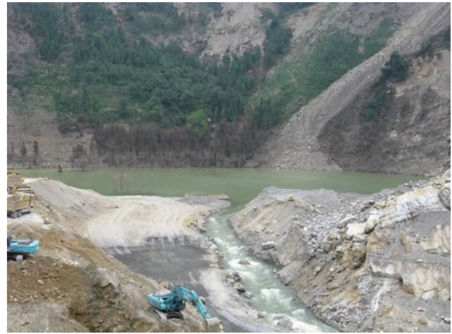
Fig. 2 The Xiaojiaqiao landslide which formed the second largest landslide dam on the Chaping River, in Anxian County. An artificial spillway was blasted and dug through the landslide dam to allow the river to resume its flow. The dead tree-line marks the elevation of the maximum level of the water, which was building up behind the dam, before the spillway was dug (Photo taken July 6, 2008, by Lynn Highland, U.S. Geological Survey)
