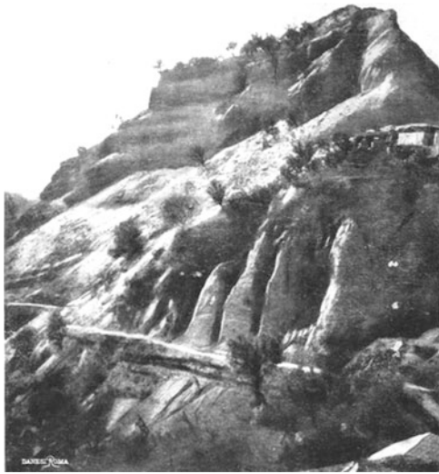
Fig. 8 The rock fall on the mule track between Cataforio and S. Salvatore (East of Reggio Calabria), that killed three muleteers (Taramelli 1909)
