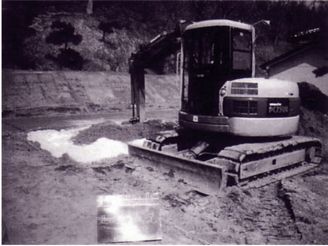
Fig. 4 Construction of surface ground improvement for house B, total of 10 t cement was mixed into the ground
