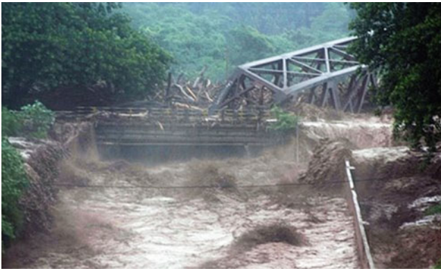
Fig. 9 Packham Avenue bridge during the flood
